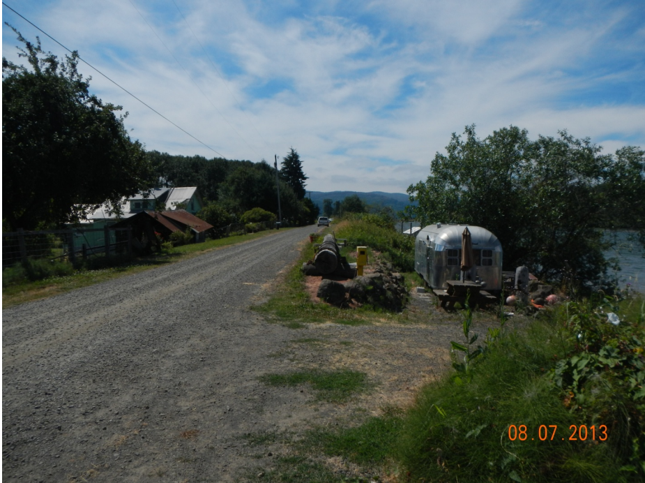
Photo 6. Encroachments into riverward levee slope including cuts into the embankment, oversteepening and unapproved construction of trailer platform.
