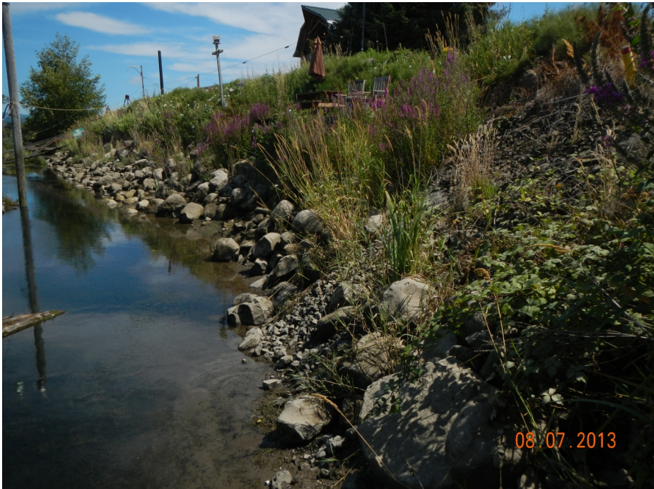
Photo 7. Encroachments into riverward levee slope including cuts into the embankment, oversteepening and unapproved platform construction.
