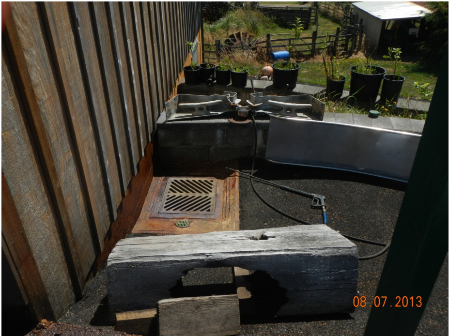
Photo 6. Surface water drainage structures of unknown construction installed within the levee prism.
