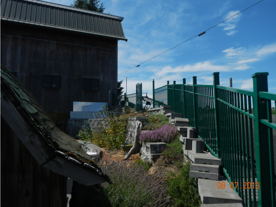
Photo 3. Encroachments including barn and terraced retaining wall construction within the landward levee prism.
