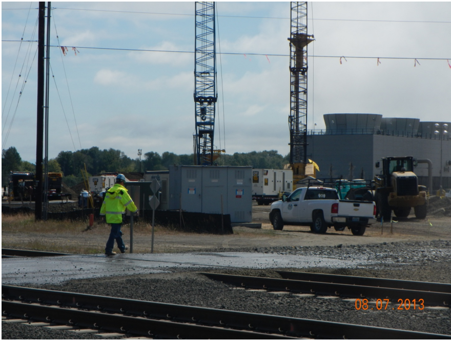
Photo 2. Construction activity and rock column installation at the PGE Port Westward Unit II site.
