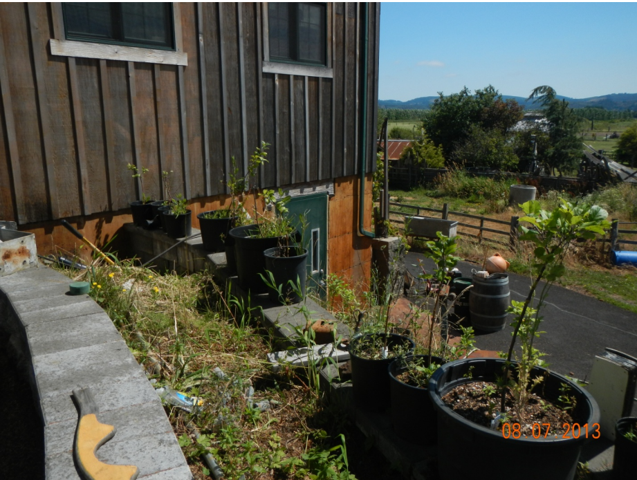
Photo 4. Encroachments including barn and terraced retaining wall construction within the landward levee prism.
